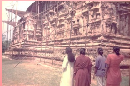
Thiwanaka image house at Polonnaruwa with a standing Buddha statue made up of bricks with three curves at knees, waist and shoulders. An outside view of image house during conservation. There are entrancing wall paintings inside with beautiful carvings outside.
