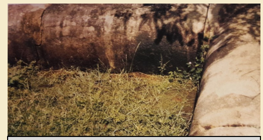
The wall made up of stone surrounding the pancāwāsa to conserve rain water
